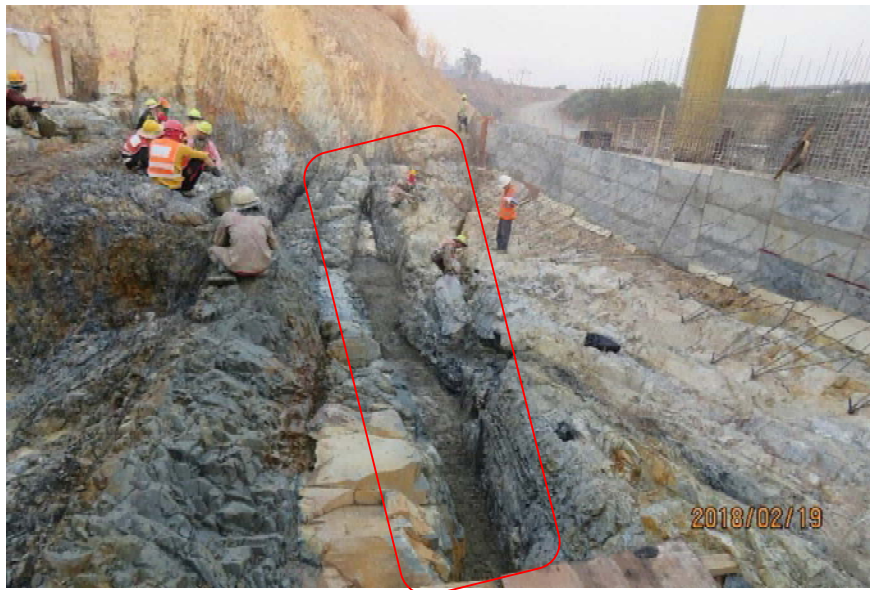
Figure 4.4-1 Crushing zone along Bedding Exposed in Excavation of Embankment 1 of first phase (as indicated in red box)
