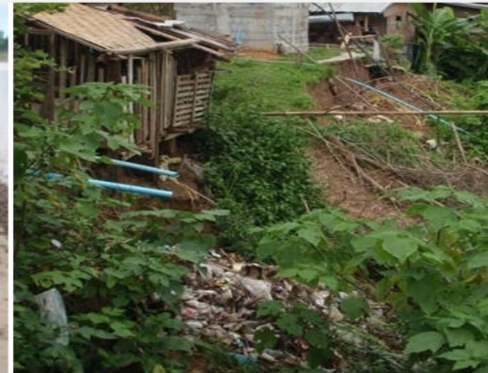
River Bank Erosion and Garbage D
