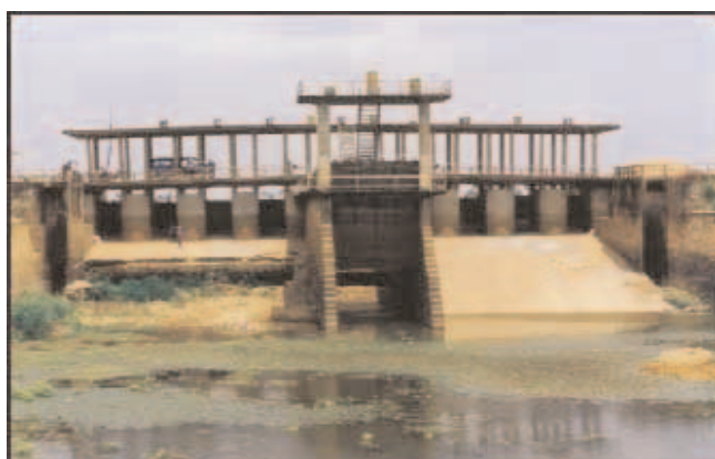
Irrigation weir on the Stung Chinit, a tributary of the Tonle Sap. Built under the Khmer Rouge, this defunct weir will soon be rehabilitated and will incorporate a fishpass for migrating fish, and a continuous release of water to the river downstream
