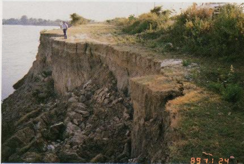
◆ Bank collapse at Sithantai near Vientiane
