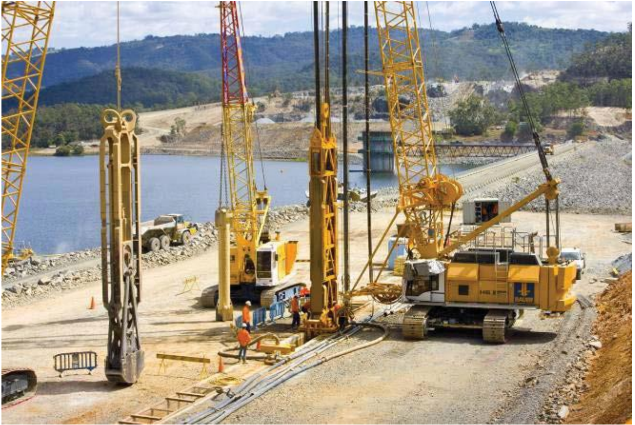
Figure 12: General view of construction of Cut-off Wall at Hinze Dam in Austria
